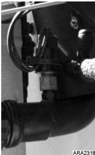
Figure 133: Low Pressure Cutout Switch Installed
