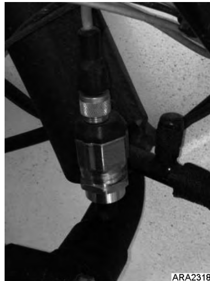
Figure 134: Suction Transducer Installed
